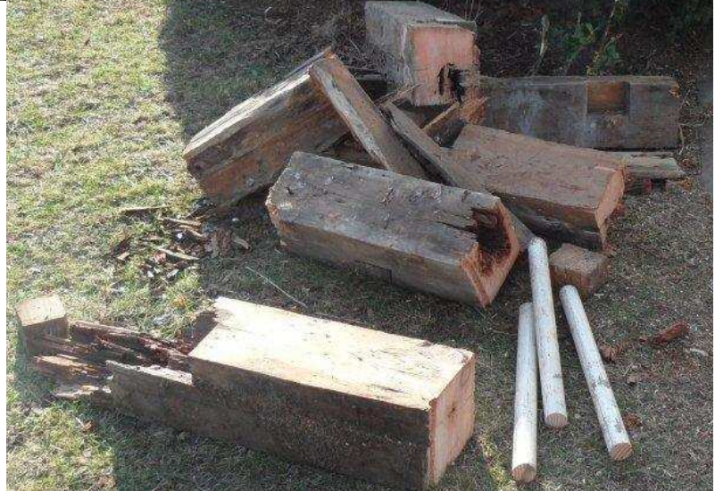
The sill removed from the church shows significant rot. Photos by Chris Laughed.
